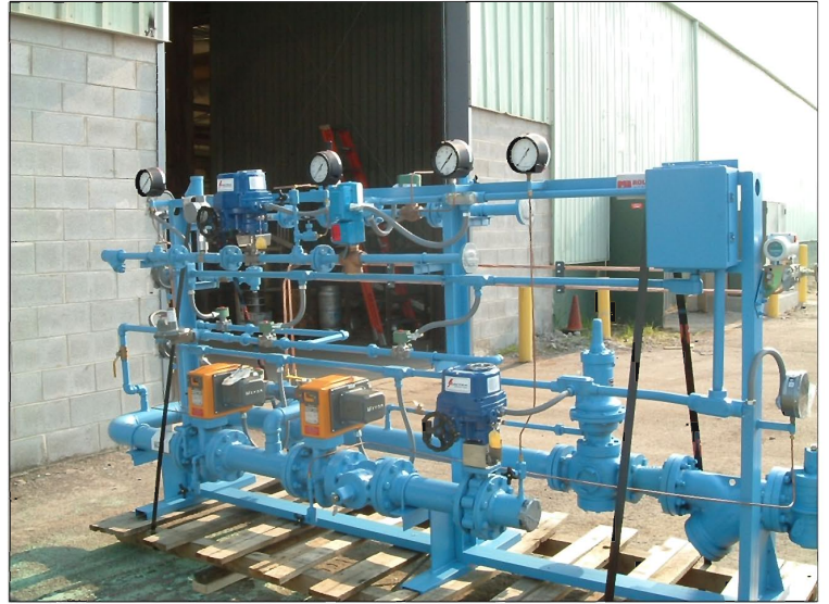
Steam pipe and control valves for industrial boiler gas burner.
